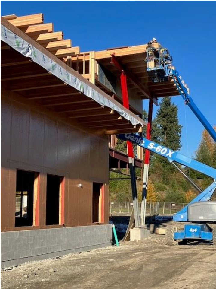
Station 111 , Main entrance and building fronting Veterans Memorial Drive. Masonry installed around the facility.
