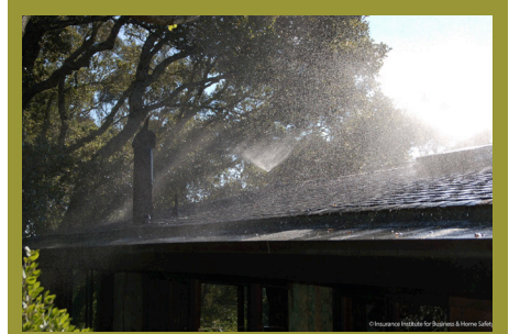
Photo 1. Roof mounted sprinkler.
