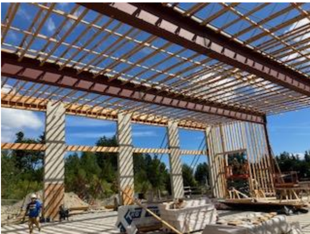
The apparatus bay slab and roof trusses. The roof sheeting will start this week.
