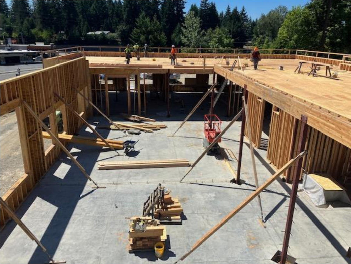
Roof deck Framing of the administration wing. Taken from the 2 nd floor operations area.
