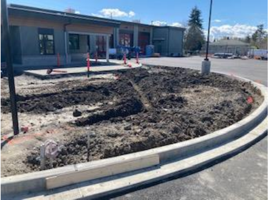
Landscape irrigation sprinkler system
