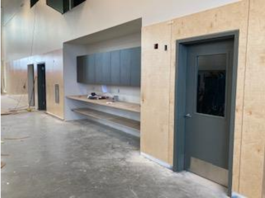
Battery charging area in the apparatus bay
