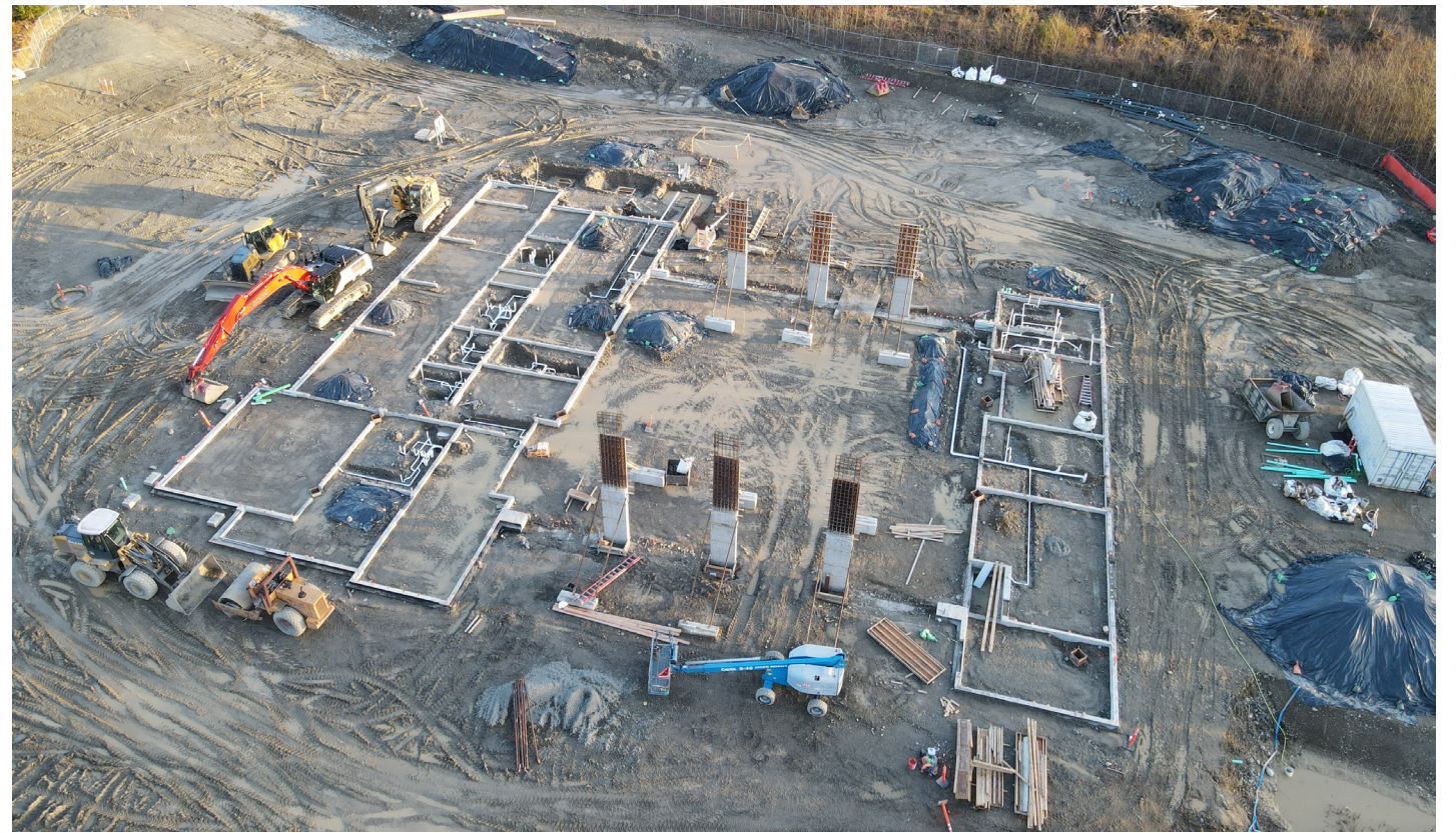
Foundation work takes shape on the new Tehaleh Station 117, slated to open in early 2025.
